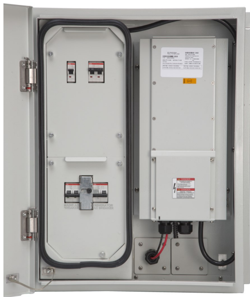
AC Input and CC1600 rectifier compartment
