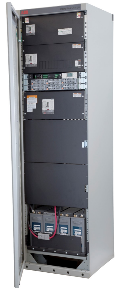
DC Power System - Type 1
