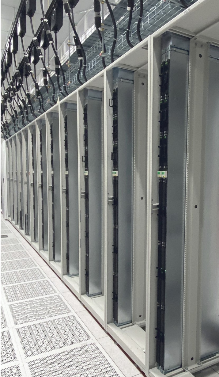
Edge Data Center Power Architecture Installation.
